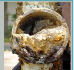
Sewer Pipe Clogged with grease
